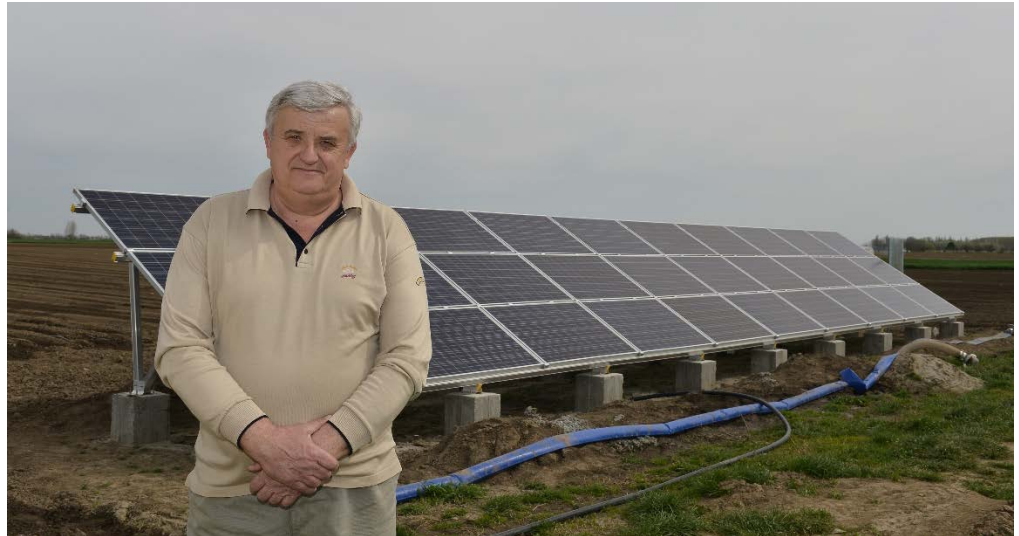
Solar-powered Irrigation Drip System in Begeč, Serbia.
