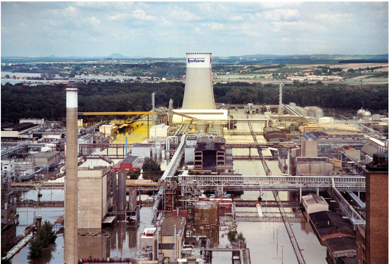
Figure 1. Chlorine release at the flooded Spolana plant. Source: © Václav Vašků.
