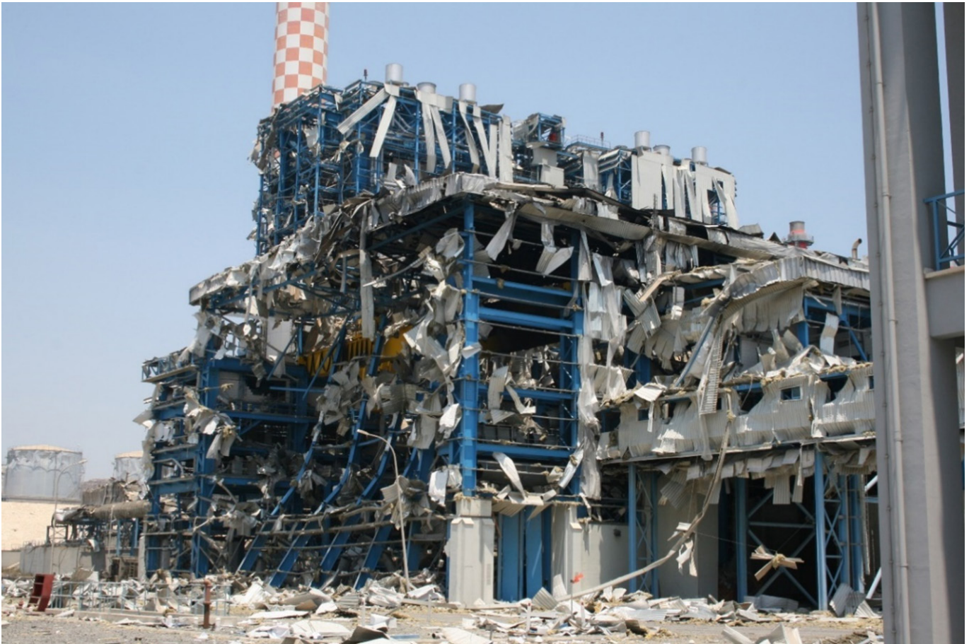
Figure 3. Vasilikos power station after the Florakis Naval Base explosion, Cyprus. Source: photo courtesy IDE Technologies Ltd.
