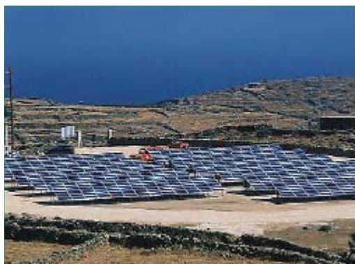
Figure 9: A 60 kWp Modular PV System on the Greek Island of Sifnos
