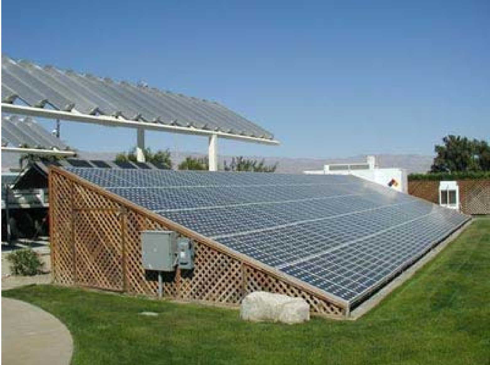
Solar panels absorb energy to produce hydrogen at SunLine Transit Agency.
