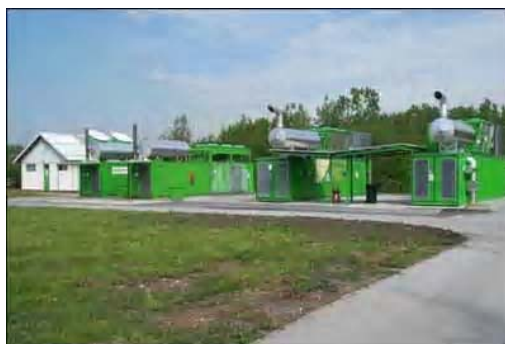
Figure 3.2: Landfill gas engines installation in Ljubljana landfill
