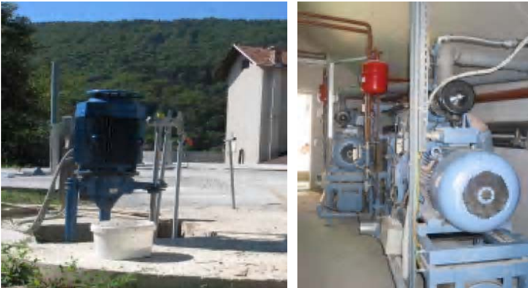
Figure 3.3: Biogas CHP installation on private farm in Letuš
