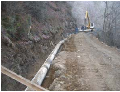
Figure 6. Steel pipeline – “underground” “underground”
