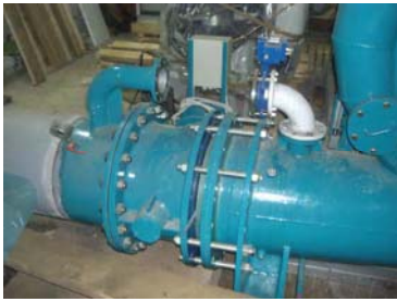
Figure 10. The lid in front of turbine
