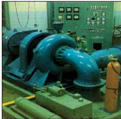
Small Hydro power house containing Francis turbine
