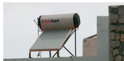
Solar thermal system for hot water heating
