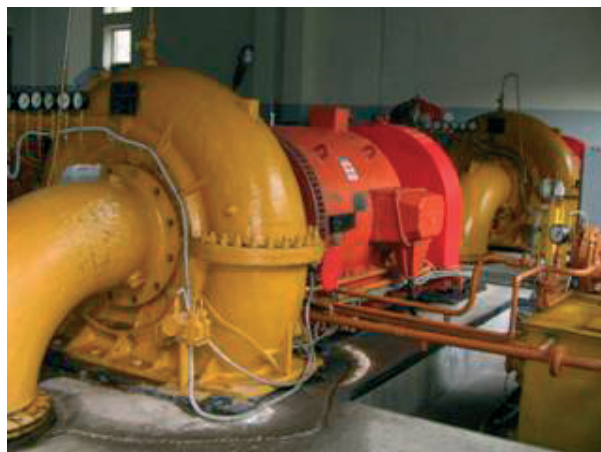
Small hydro power station
