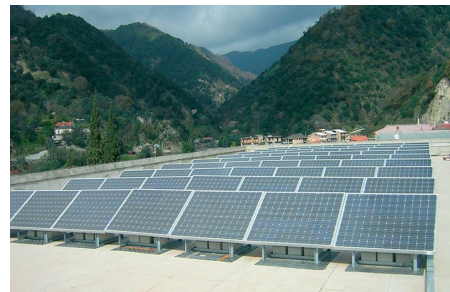
Central PV system
